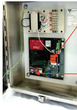
Receiver in NEMA 4 Enclosure
